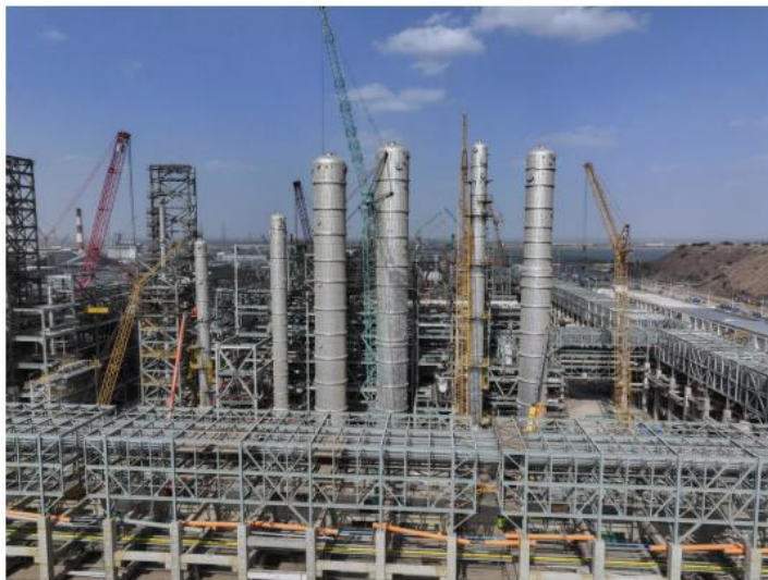
Hydrochlorination Distillation Columns
